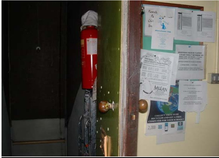
Fig 3. Asbestos Strip to Old Fire Door.
