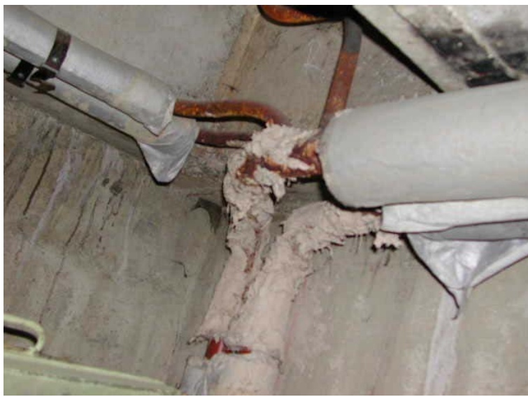
Fig 7: Asbestos Insulation on Pipe Work.
