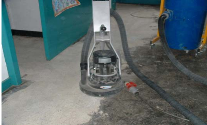
Fig 1: Asbestos containing adhesive to floor tiles.
